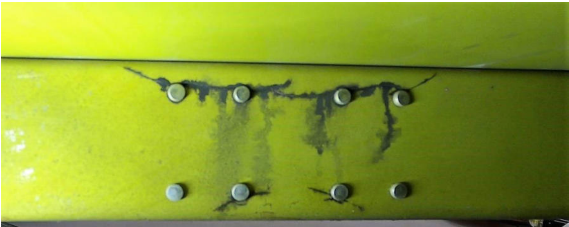
FIGURE 2 - EXAMPLE 1 - CRACK LOCATIONS - FWD SIDE OF SPAR
