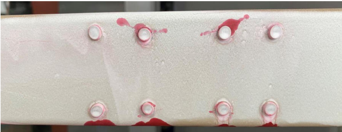
FIGURE 4 - EXAMPLE 2 - CRACK LOCATIONS - FWD SIDE OF SPAR
