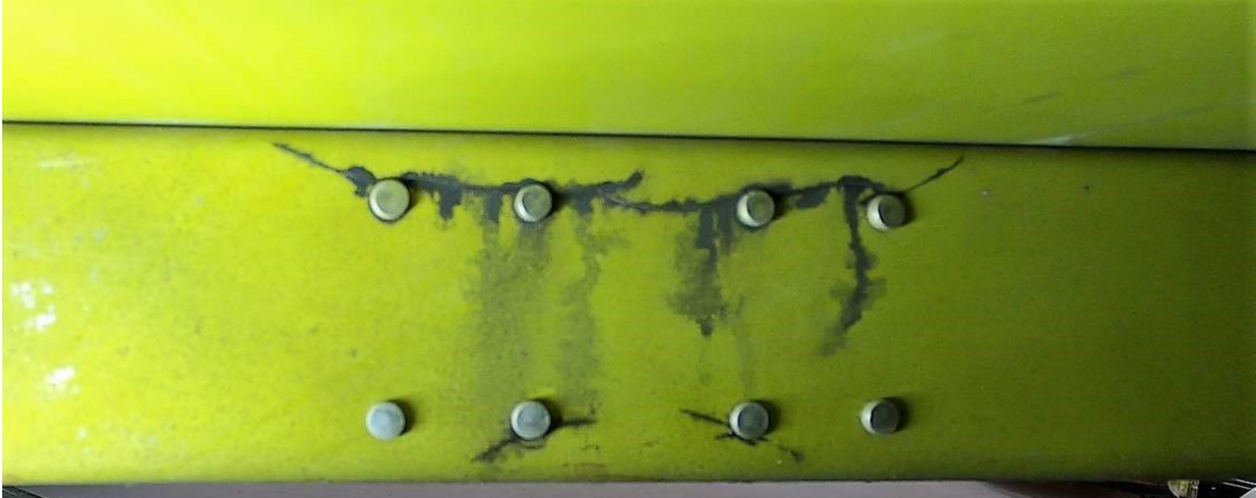
FIGURE 2: EXAMPLE 1 - CRACK LOCATIONS - FWD SIDE OF SPAR
